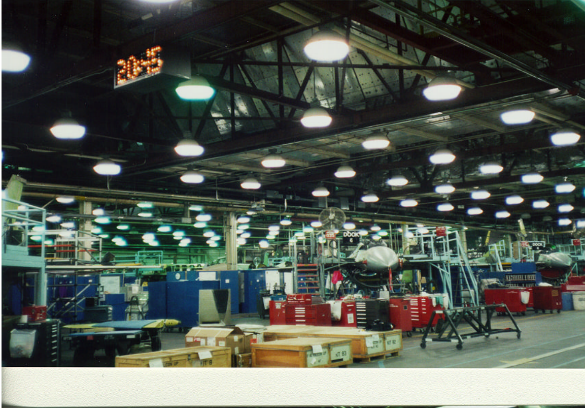
Figure 6. Post Retrofit Illuminance (fc) at 30" from floor in Dock 45 (F16) w/equipment moved away (filled data)
