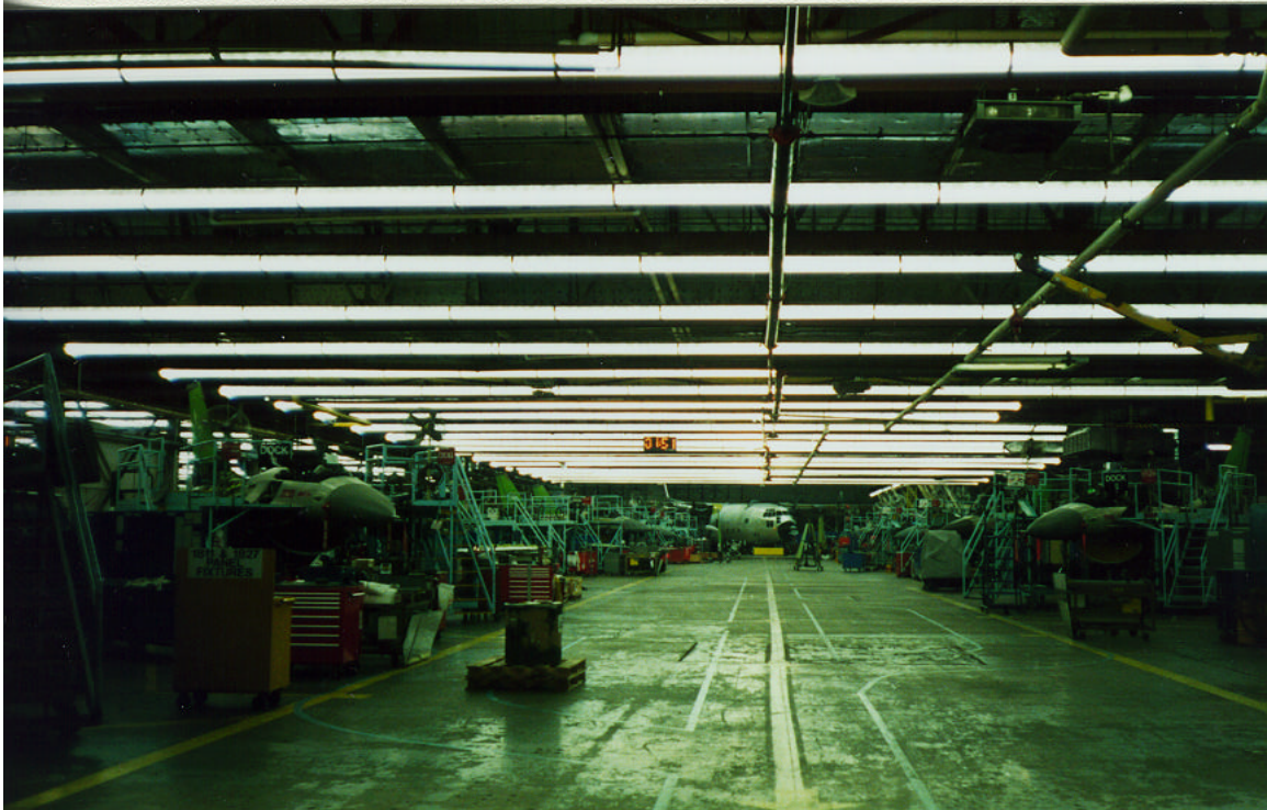
Figure 8. Pre- (top) and Post- (bottom) Retrofit Lighting Systems Down Main Aisle.
